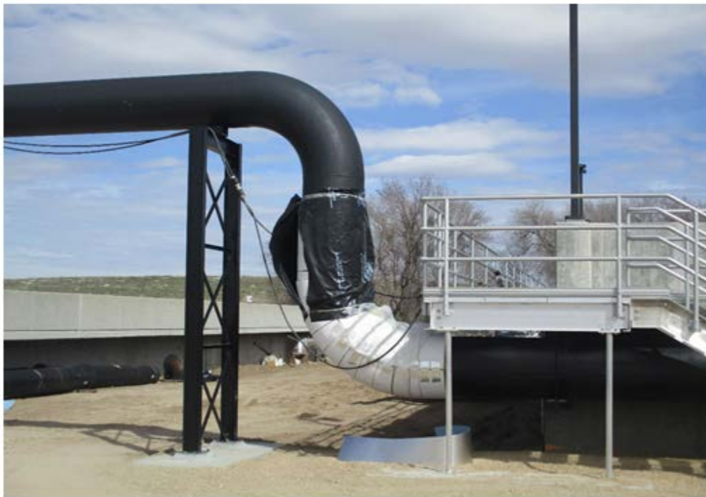
Figure 1 – Air pressure line connection to Aeration Basin No. 3
